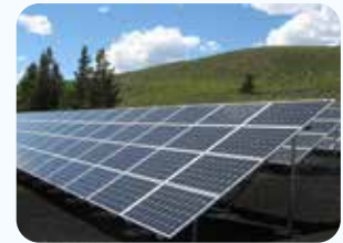
Solar energy, Power solar panels
